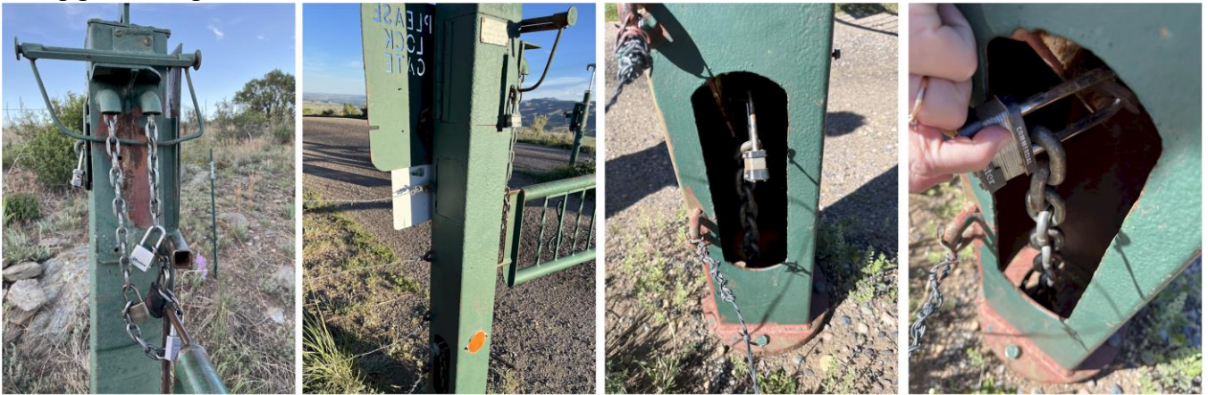
Chain closure on west face of post with authorized locks
