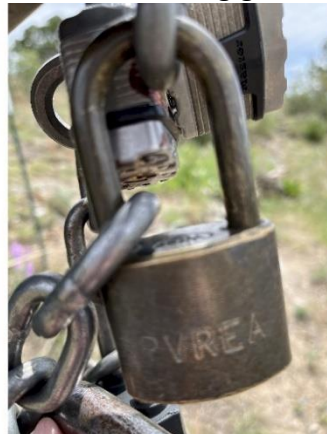
Poudre Valley Rural Electric Association PVREA Keyed Lock
